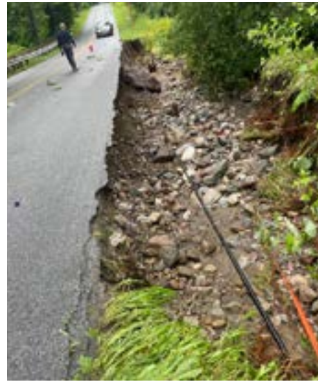
Selectboard chair Jim Faulkner examines damage on State Park Road.
