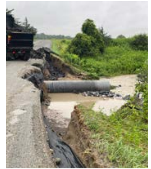
East Thompson's Point Road is back to two lanes after extensive work to repair the areas where it had become dangerous to drive near the side.
